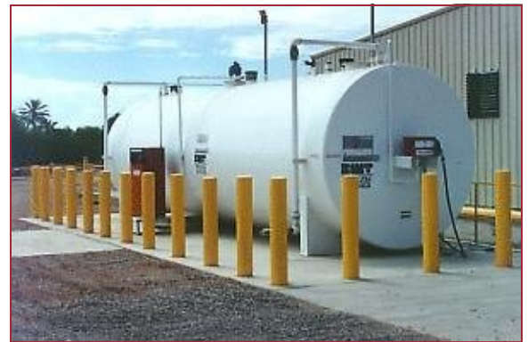
1 - Above Ground Storage Tank
